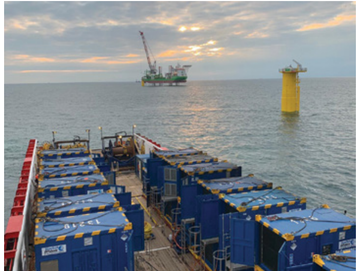
(top) A noise mitigating bubble curtain created around a wind farm monopile and (below) ScanTech Offshore air compressors lined up and ready for action
